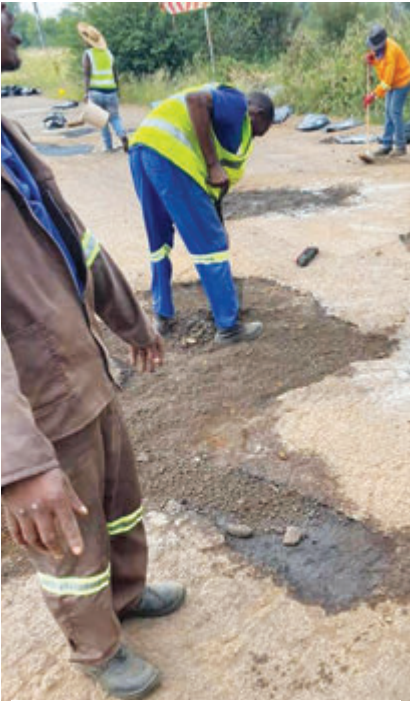
TLM personnel fixed up potholes early in the year. This reader is requesting the municipality to also attend to other roads in Northam.
